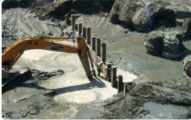
Groundwater inflow degrades concrete quality
