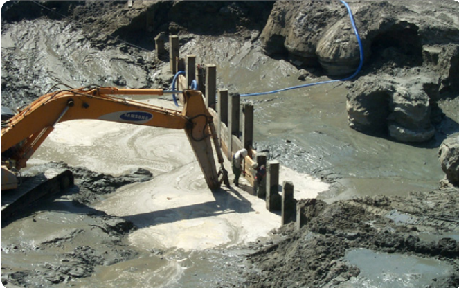
Groundwater inflow degrades concrete quality
